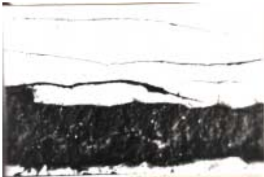
Fig 2. Picture of typical finishing surface destruction of glazed ceramic tile
