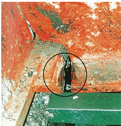
Figure 2. Fracture at beam-column-connection of the steel structure damaged by Kobe earthquake in 1995
