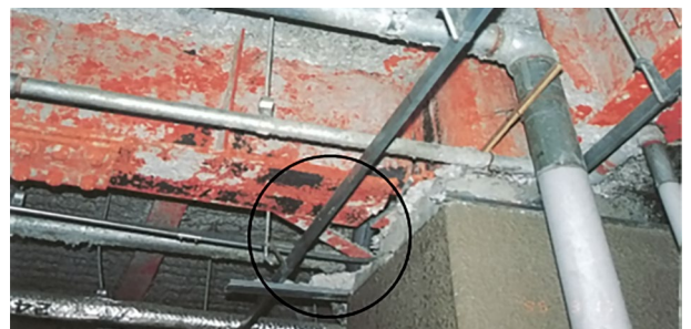
Figure 1. Steel structure damaged by Kobe earthquake in 1995
