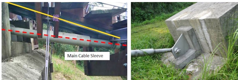
Figure 3. Pictures taken at anchorage of main cable (left) and stabilizing cable (right)
