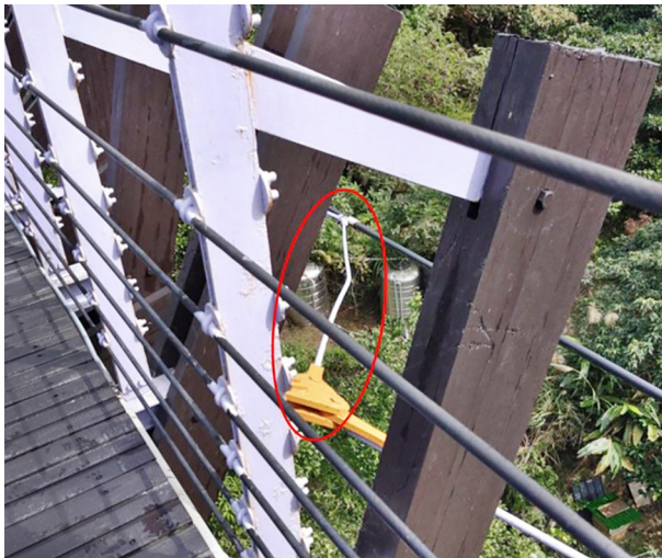
Figure 4. One of the buckled and rusted steel connecting rods
