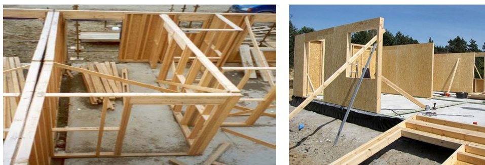
Fig. 4. Building constructed in the line system and in the large panel technology
